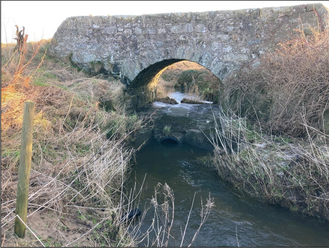
Photograph 2: Burn of Boyndie (WC02), Culvert at d/s end of the Survey Extent.
